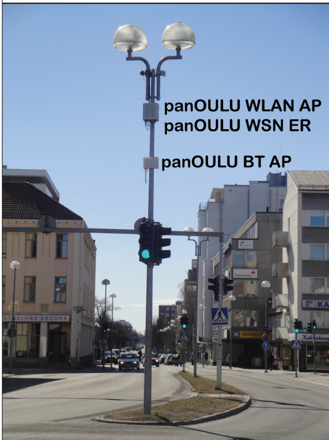
Figure 2. A panOULU wireless LAN access point (WLAN AP), wireless sensor network edge router (WSN ER), and Bluetooth access point (BT AP).
